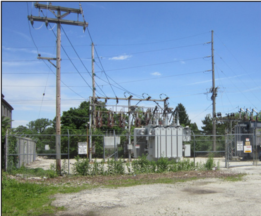
ComEd substation located southeast of the Metra station.
